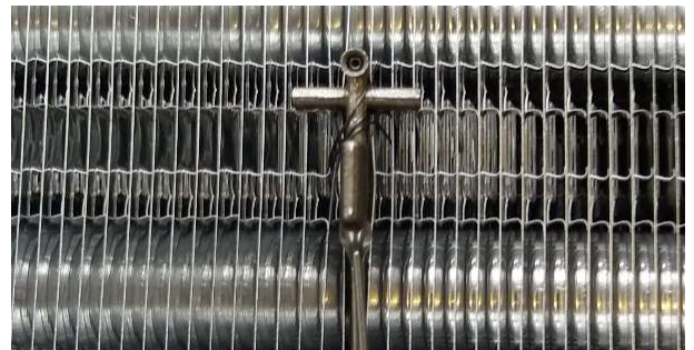
Figure 2 Probe (S_KPS_qxpkjf) mounted on radiator.
